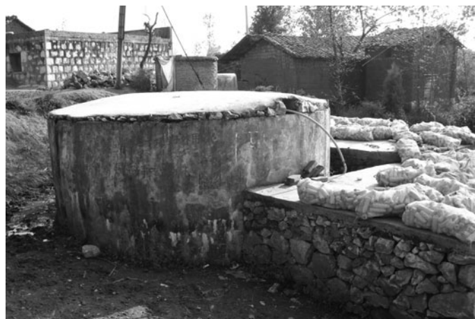
Rainwater collection tank
