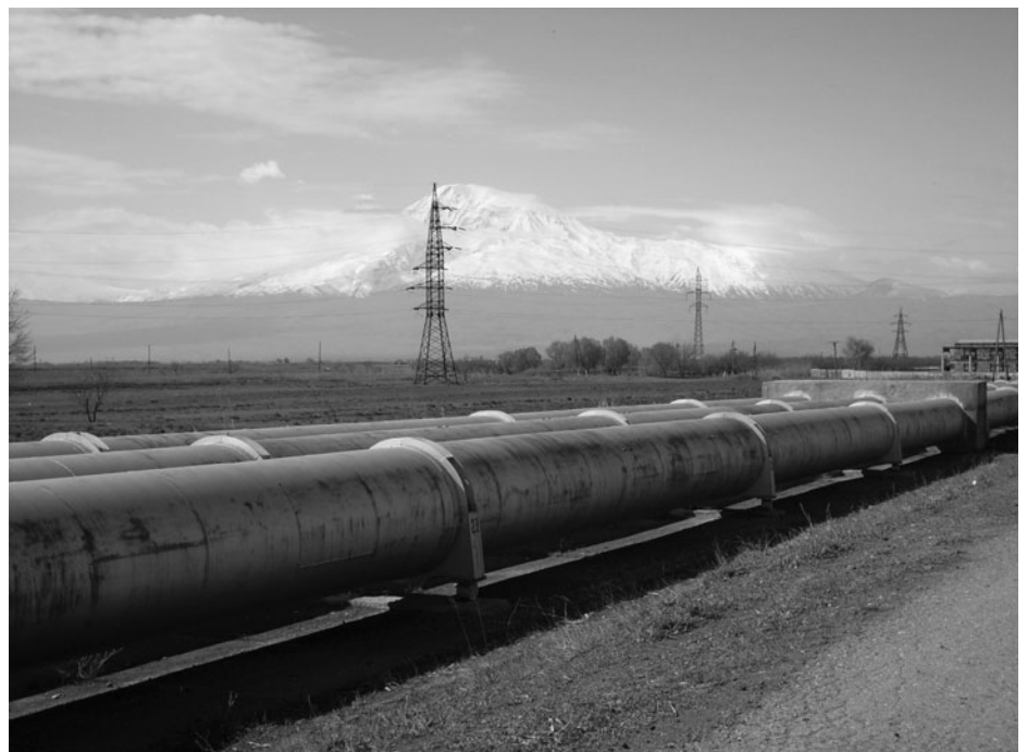
Pressure pipeline in project area
