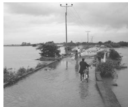
Sri Lanka: Heavily damaged Kiran Causeway
