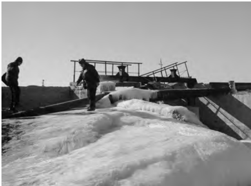
Kazakhstan: Wearying ice – leaking transmission main at 20 degree below zero
