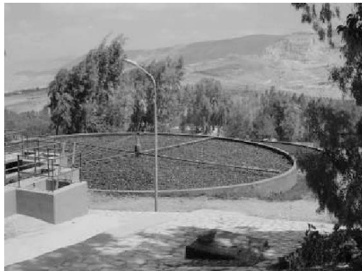
JORDAN: Trickling Filter at a Waste Water Treatment Plant
